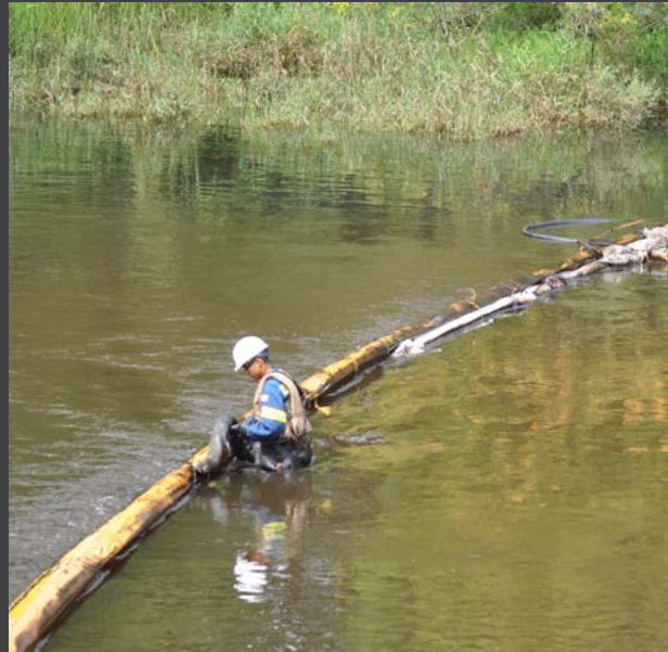
WORKER CLEANING UP AFTER THE KALAMAZOO RIVER SPILL.
